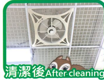
清潔前 Before cleaning
